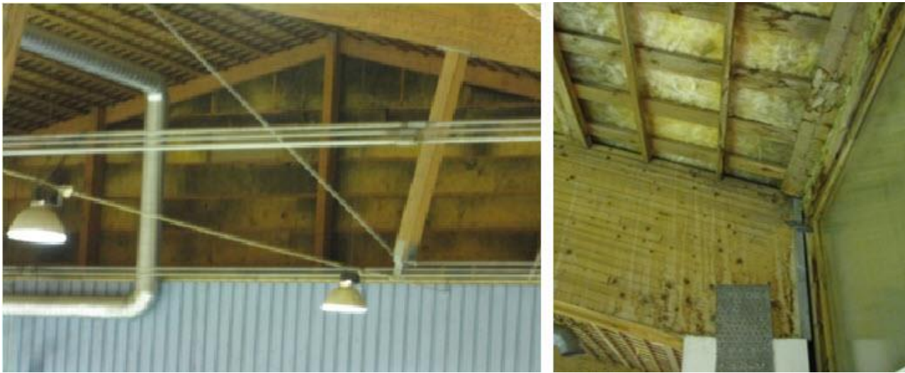
Figure 22 Mould on and in in wall structures.
