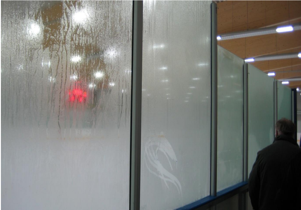
Figure 3 A common symptom of too high humidity in an ice rink.
