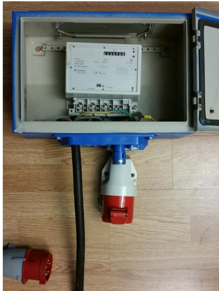
Figure 36. Electricity meter with 32 A connectors
