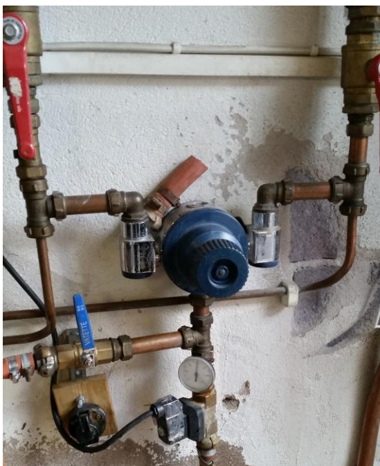
Figure 29. Water system with water mixed before valve in one of the examined ice rinks
