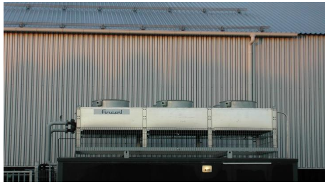
Figure 17. Dry cooler in a Swedish ice rink
