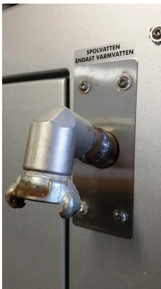
Figure 24. Resurfacing machine water tank inlet marked with "Only hot water"
