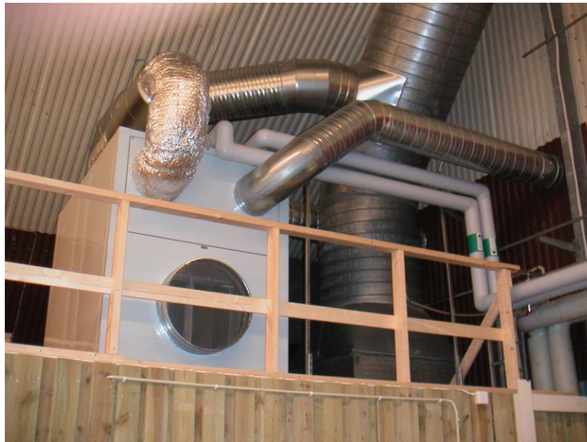
Figure 7. Desiccant humidification system connected to the ventilation system in a Swedish ice rink
