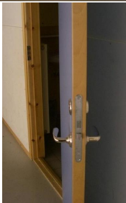
Figure 11. T.V. Open toilet doors towards the ice rink's arena room. T. H. Non-insulated doors are not suitable for separating climate zones.
