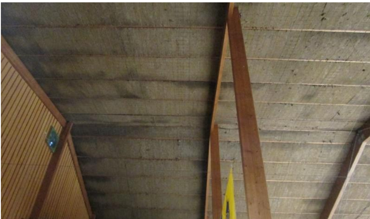
Figure 2. Traces of air leakage between wall and ceiling.
