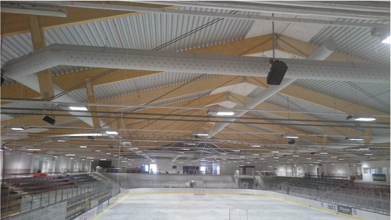
Figure 20. Textile channel for both ventilation and dehumidification in an ice rink.
