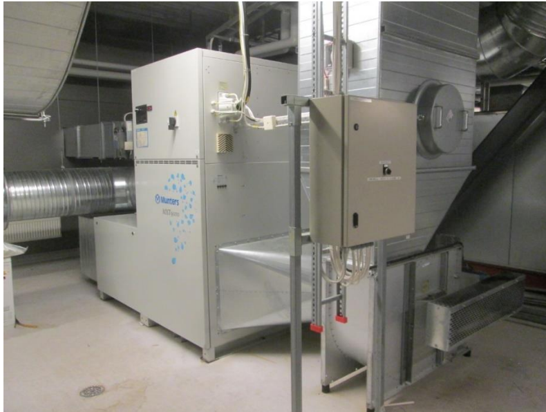
Figure 3. A larger desiccant dehumidifier in a Swedish arena facility.
