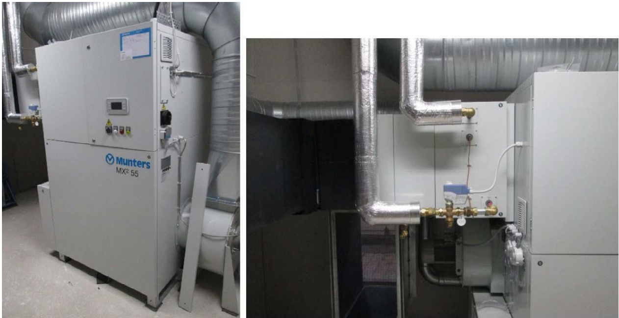
Figure 12. First generation hybrid dehumidifier (TV) - the connection to the heat recovery (TH).
